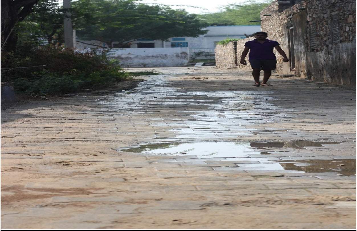
Un-proper drainage in Asarwa village.
